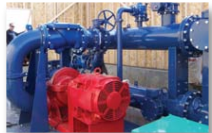
Horizontal pump station
