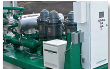
Vertical pump station
